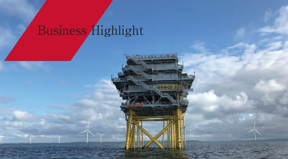
Offshore wind substation
